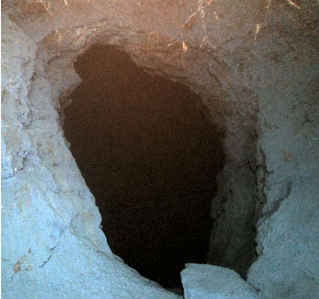
Plate 18: The hole in the main chamber wall at PS11B that leads into the PS8 'side pipe working' entered from the pumping shaft
