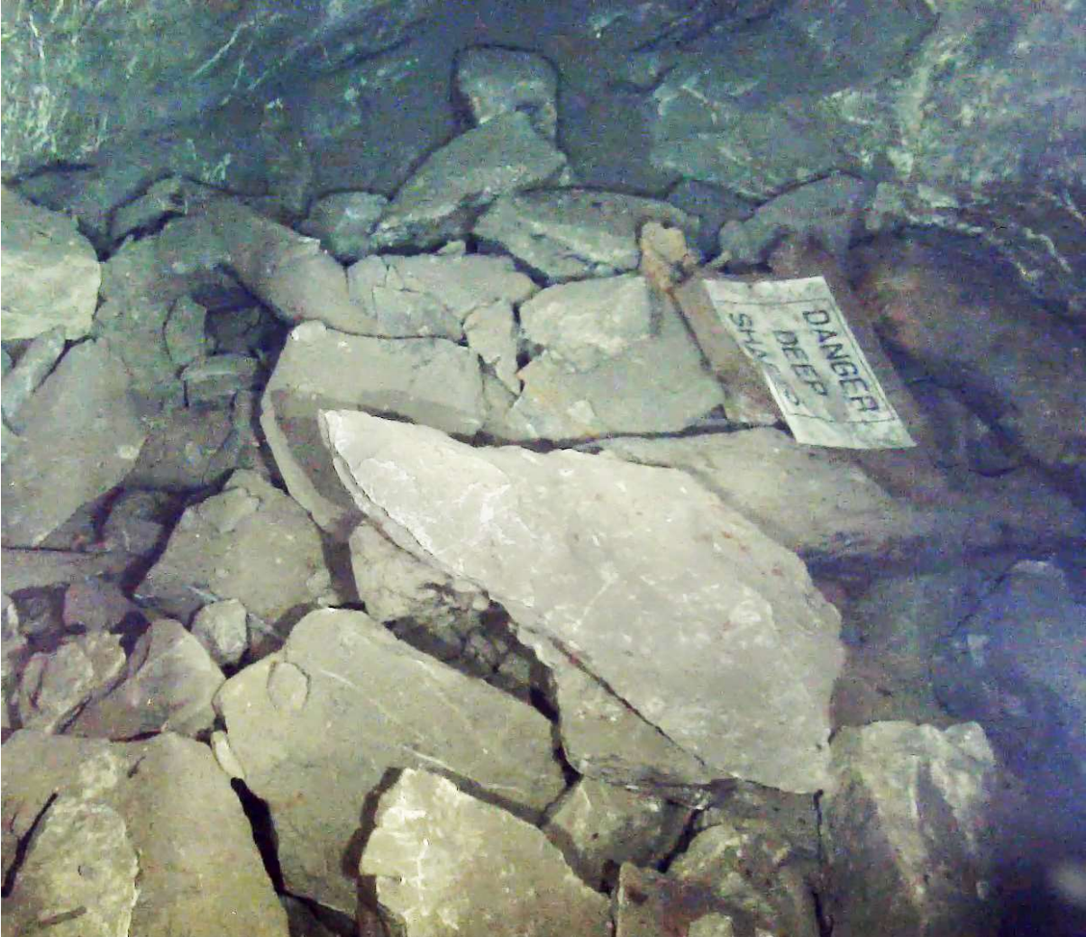
Plate 23: The rubble at the present NW6 base of the North Winze, presumed to have been thrown down in the 1790s after the trial using the shaft was abandoned. The danger sign only came down the shaft recently after it became detached from the modern safety chain at the shaft top
