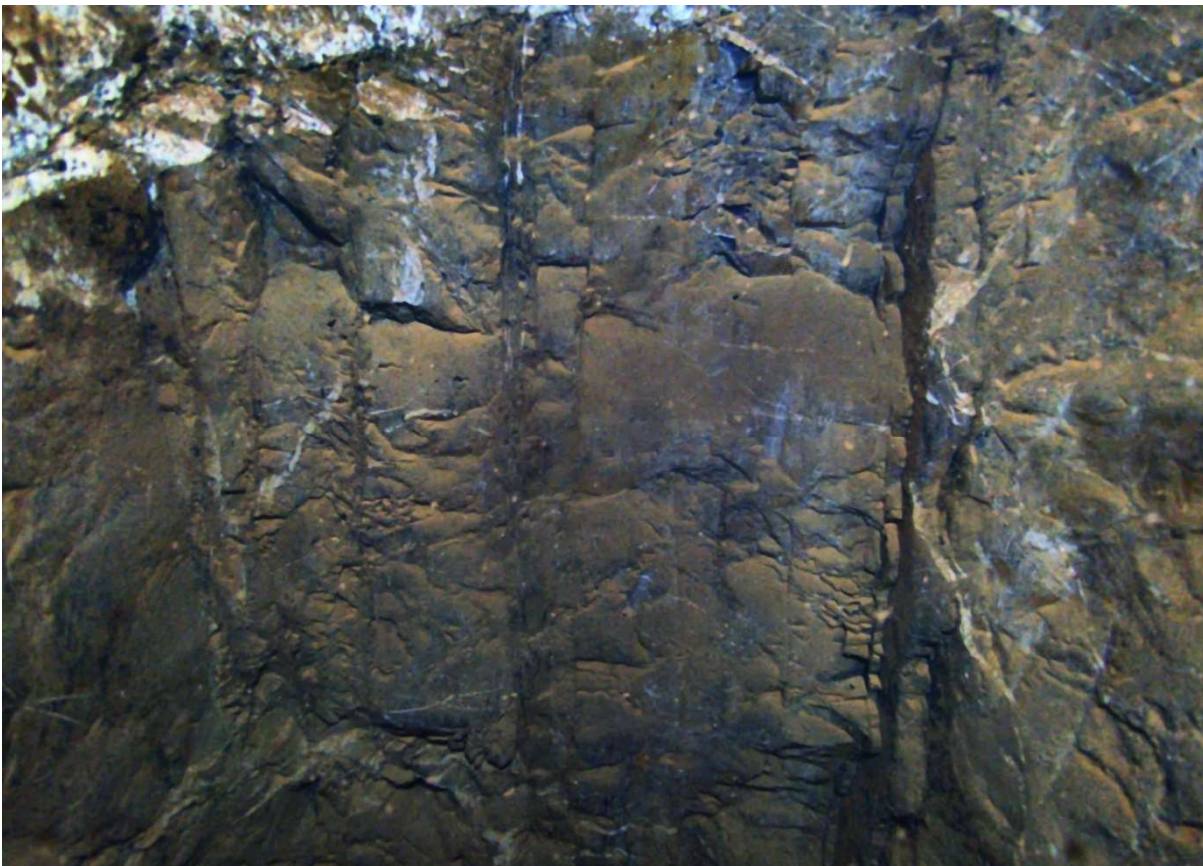
Plate 4 Thickly bedded limestone in the winding shaft at c. -36.5 down, with the dip near-vertical because of folding
