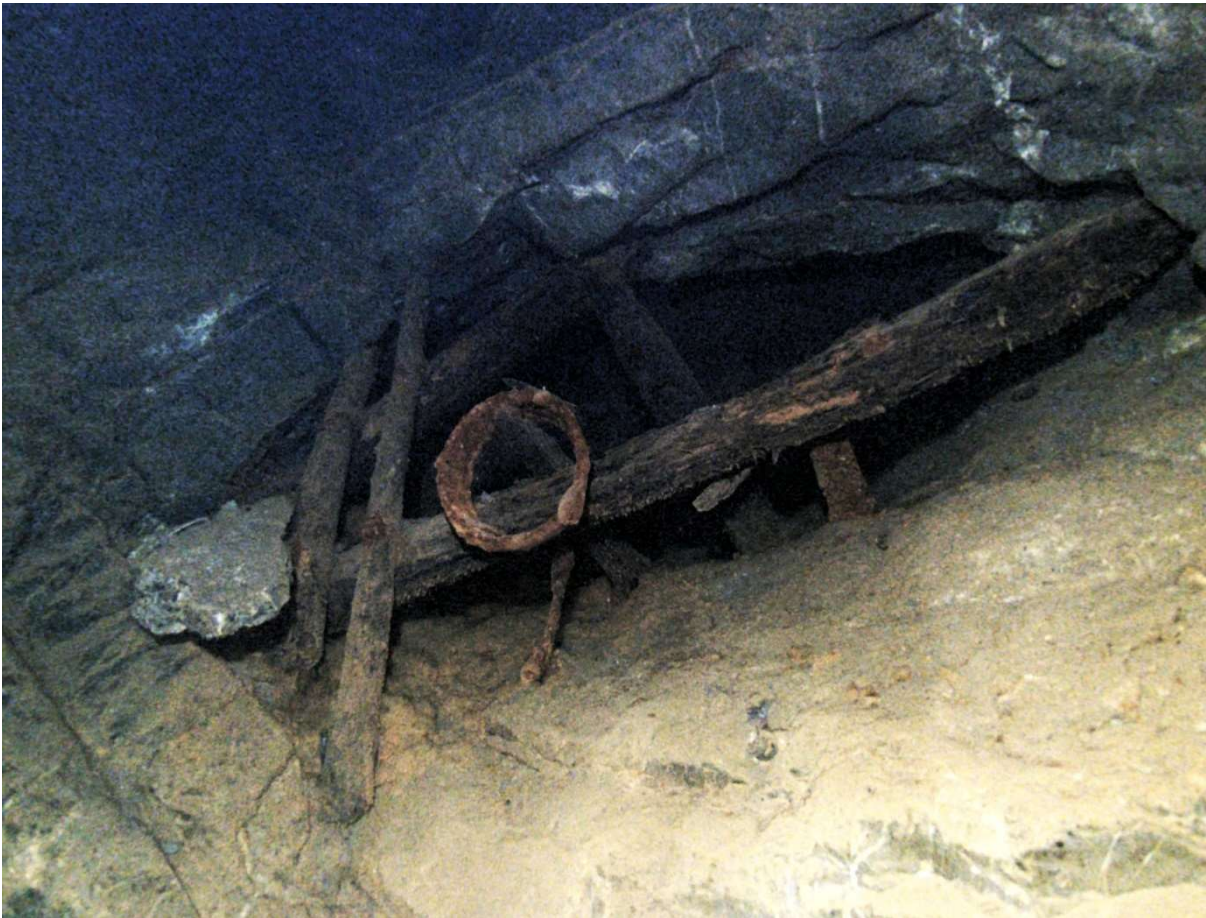
Plate 13: Looking diagonally upwards into the entrance of the 'side pipe working' at WS6 in the winding shaft, with a collection of timbers, some at least of which have collapsed downwards from within the working. The metal ring was placed here after the collapse
