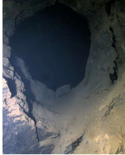
Plate 19: The hole in the main chamber wall at PS11B as seen from the other side where it is high in 'side pipe working' entered from the pumping shaft (PS8)
