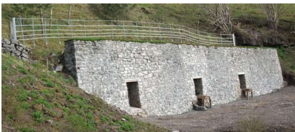
Figure 8 Restoration of the Ecton Mine dressing floor wall following detailed archaeological investigations, as restored in 2016 with financial support from Historic England
