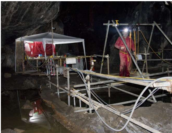
Figure 10. The launch platform, and the adjacent work station, at the pumping shaft, photographed as their installation was being completed ( Point size? )
