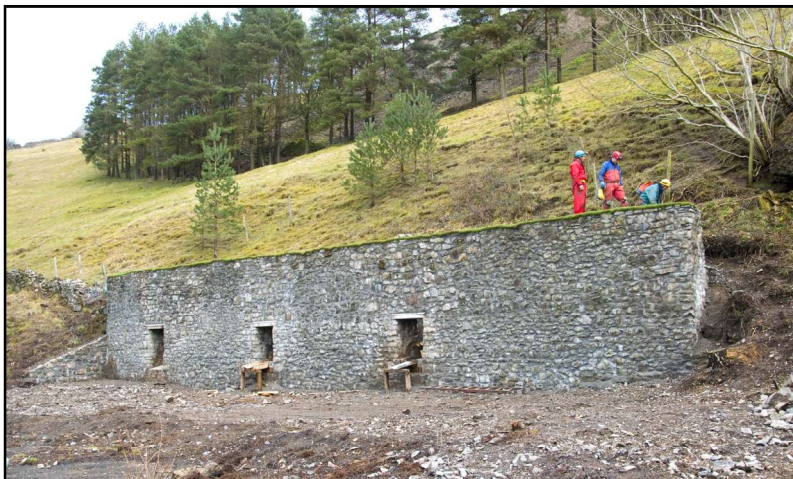
Plate 12: The dressing shed back wall shortly after restoration was completed, being inspected by members of a party who had just been in Deep Ecton Mine.
