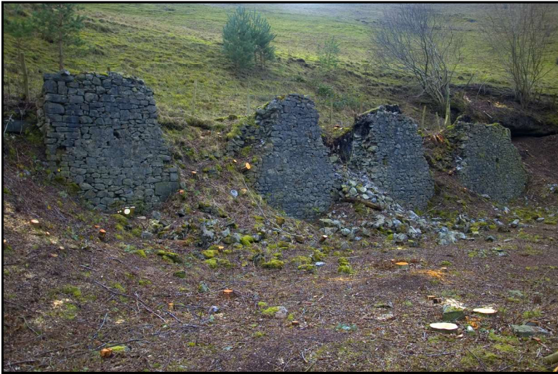
Plate 1: The dressing shed back wall in 2015, shortly before conservation and rebuilding work started.
