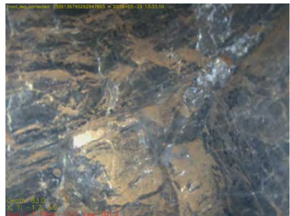
Figure 9.18: Anticline and fault (-83.0m Winding Shaft).
