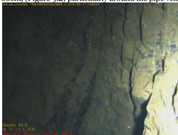
Figure 9.1: Near vertical bedding of thickly bedded Ecton Limestones (-40.6m in Great Shaft).
