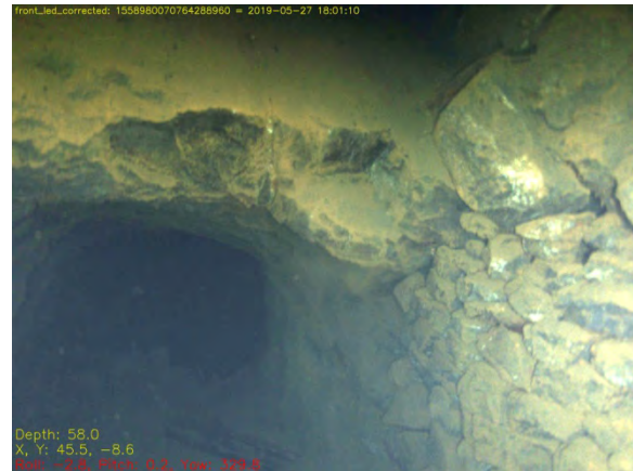
Fig. 7.55: The PW10 cross-cut to the winding shaft, with the retaining wall PW8 to the right that was built to keep the passage clear of rubble coming down the steep slope of PW6 from above.
