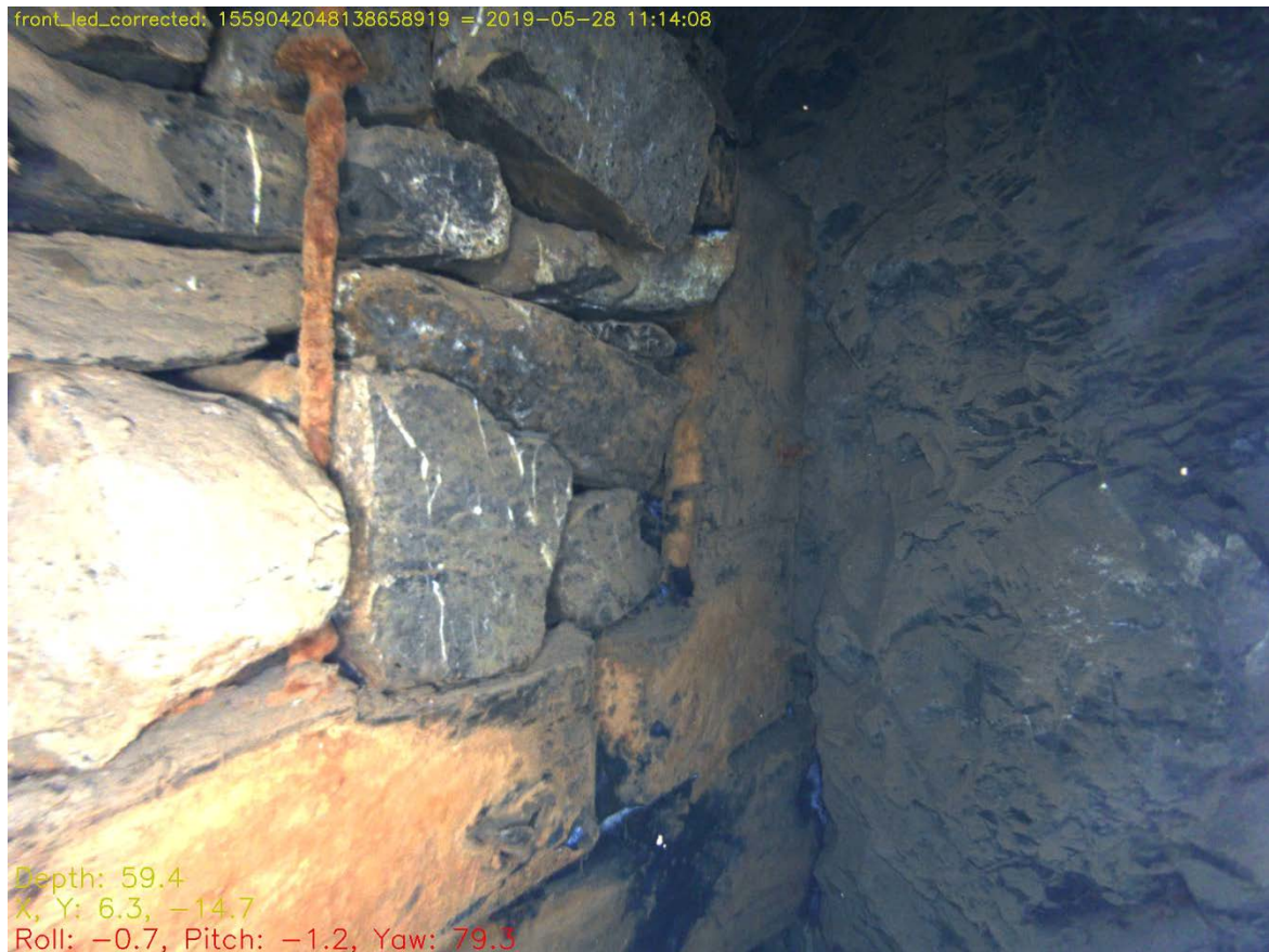
Fig. 7.33: Part of the complex arrangement of timbers above two support beams outside the base of the passage at PS9 at the south-eastern end of the pumping shaft. One of these support beams is just visible at the bottom of the photograph, with further timbers above, including a panel of planks near the shaft wall. The long iron pin was presumably also placed here to help support the crude stone wall that retains the backfilled part of the passage.
