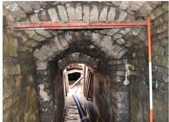
Fig. 7.5: The entrance section of the Deep Ecton Level, just above the river level, showing the October-November 2018 repairs in progress (Photograph: John Barnatt).
