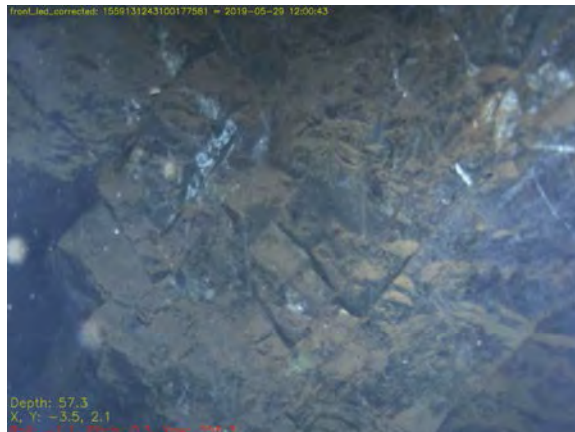
Figure 9.29: Open joints (-57.3m Winding Shaft).
