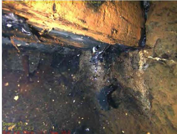
Fig. 7.28: The base of the timber platform below the level or ‘side pipe working’ at PS9, with both supporting beams visible, lies at the south-east end of the pumping shaft. Directly above these two beams there is a complex series of timbers and ironwork that hold back the rubble in this part-backfilled passage.
