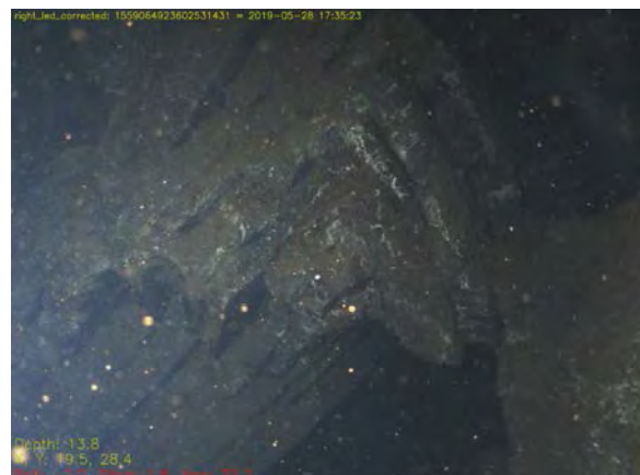
Figure 9.52: 'Saddle' workings in pipe wall - one of Watson's 'huckle saddles'? (-13.8m Pipe).
