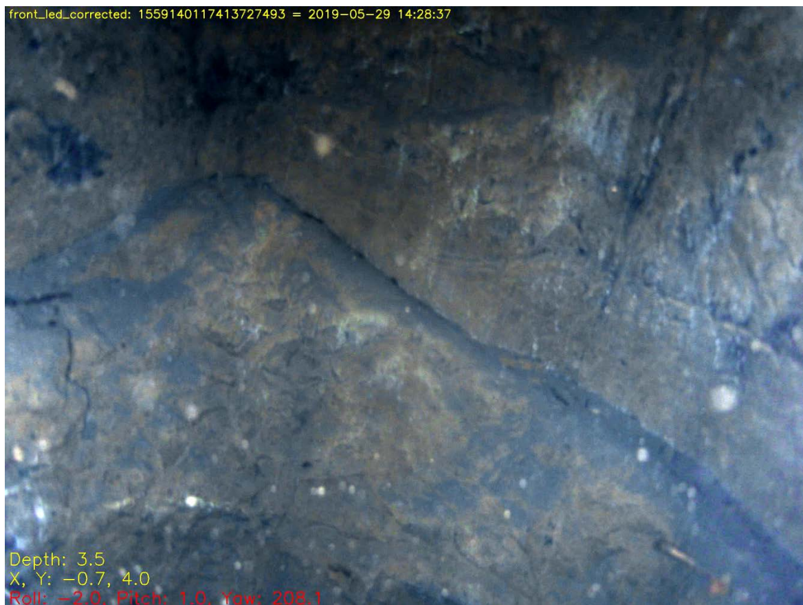
Fig. 7.43: The apex of the ‘garland’ in the winding shaft walls above the level at WS1. This small cut-channel was made to capture water running down the shaft sides and take it away via the level. Thus, it helped keep the hemp winding ropes dry, which was important because long wet ropes were significantly heavier and thus put more load on the winding engine.
