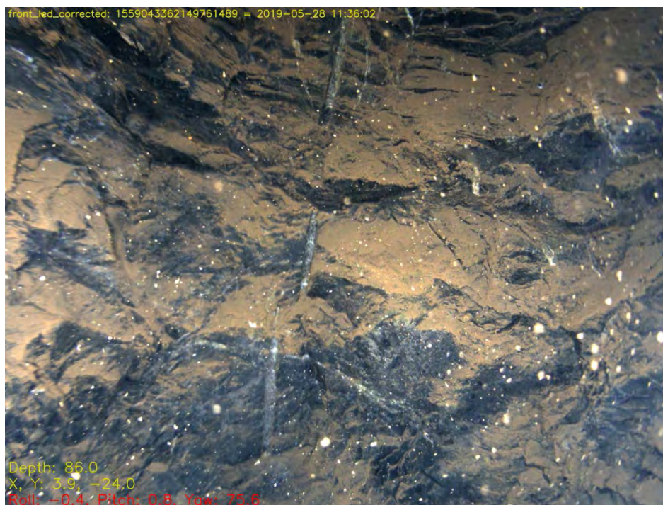
Fig. 7.19: A detail of the pumping shaft wall at -86m, showing three downward-pointing gunpowder shot hole-scars placed at regular intervals, which date to when the shaft was being sunk in the early 1780s.
