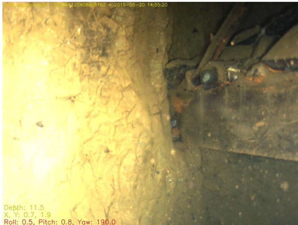
Fig. 7.32: One end of the outer timber at the PS4 platform at the north-western end of the pumping shaft; the end of the visible timber has been placed in a rectangular notch cut into the shaft wall.
