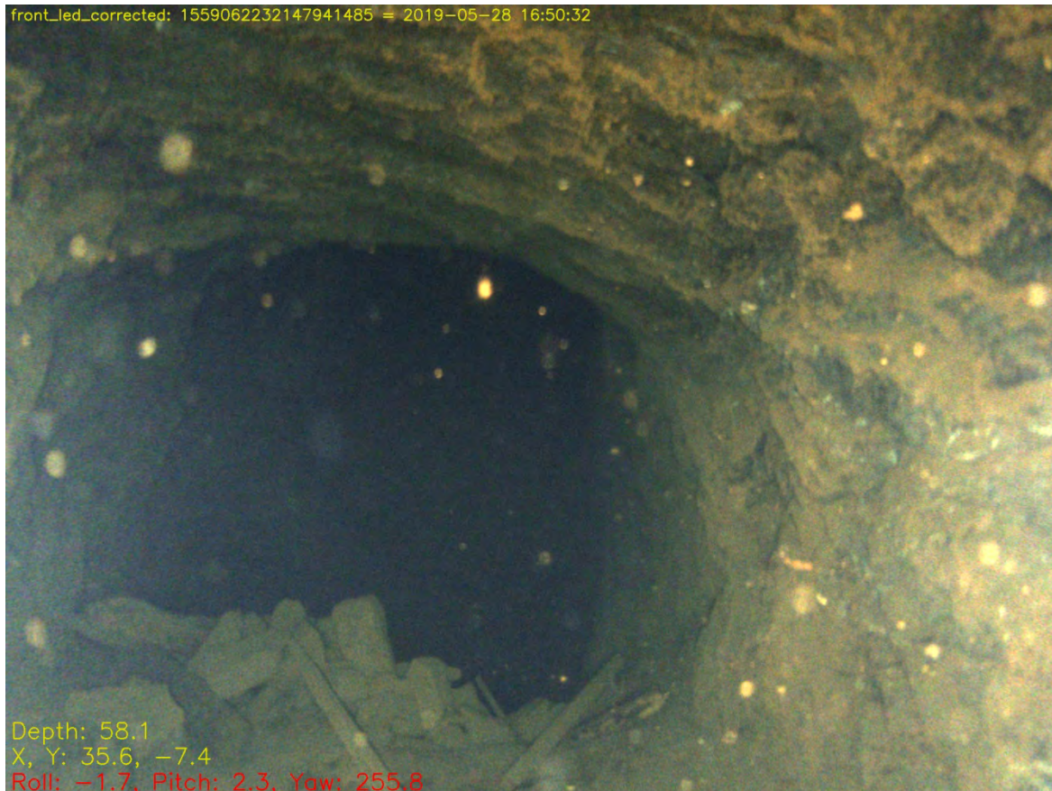
Fig. 7.57: The short -58.5m cross-cut (PW10) between the ‘main pipe workings’ and the winding shaft (PW10). The pile of rubble on the floor contains displaced timbers and a metal tramway rail.
