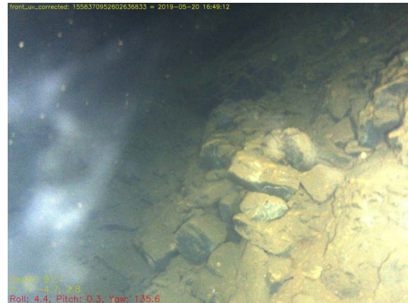
Fig. 7.22: In the large ‘side pipe working’ at PS15, in its upper part, there is an ascending slope of rubble to the right hand side, and also at the back, both visible in the gloom; visibility was not good enough to see into the area to the left how far back and upwards the working extends.
