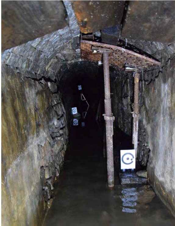
Fig. 7.4: The entrance section of the Deep Ecton Level, just above the river level, photographed in Summer 2019, showing the 1980s remedial work, and the recent bulge on one of the walls, before they were removed (Photograph: John Barnatt).
