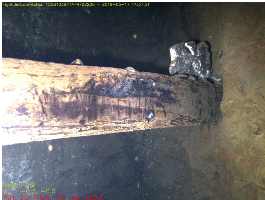
Fig. 7.30: One end of the timber at PS1 at the north-west end of the pumping shaft, showing that it is set into a carefully cut notch in the shaft wall; the shaft-end compartment for the ‘ rising main ’ iron pipes lies behind the timber to the left.
