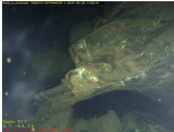
Fig. 7.21: At the base of ‘side-pipe working’ PS8, to the right-hand side, there is a separate passage at PS9 that the videos suggest is not interlinked; however, no clear view beyond was available to determine whether this was a level of a further ‘side pipe working’.
