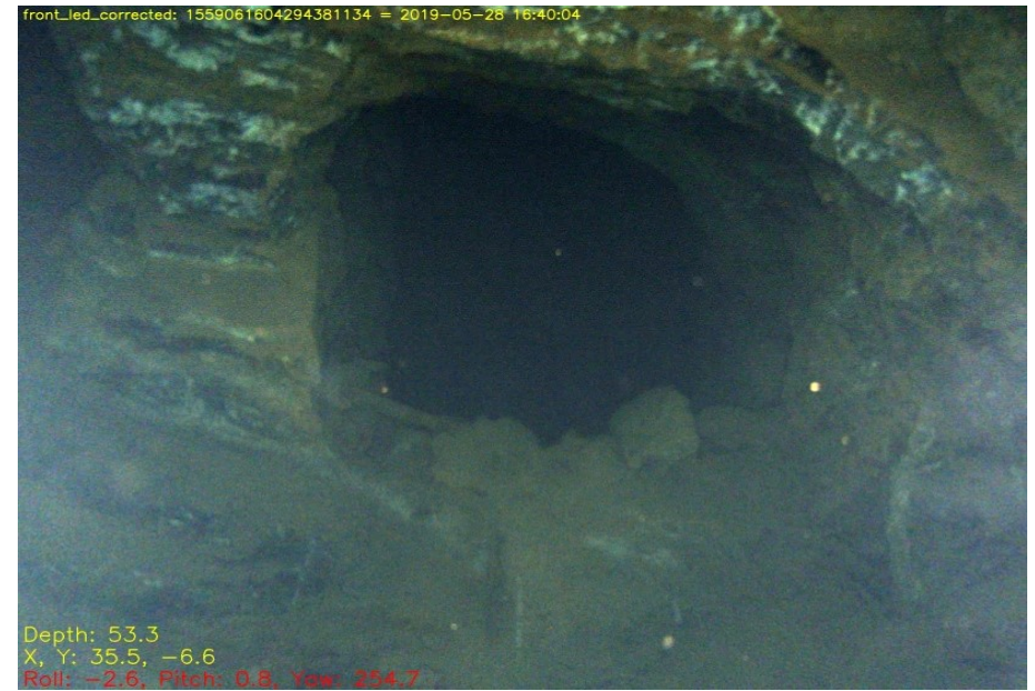
“Window” from pipe working into winding shaft at 53m depth, possibly accidental
